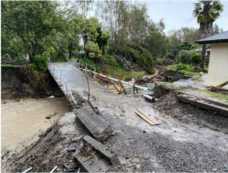
Figure 5.1- Private bridge crossing at 78 Joll Rd following the cyclone. Note the slump on the right bank and severe scour on left bank.
