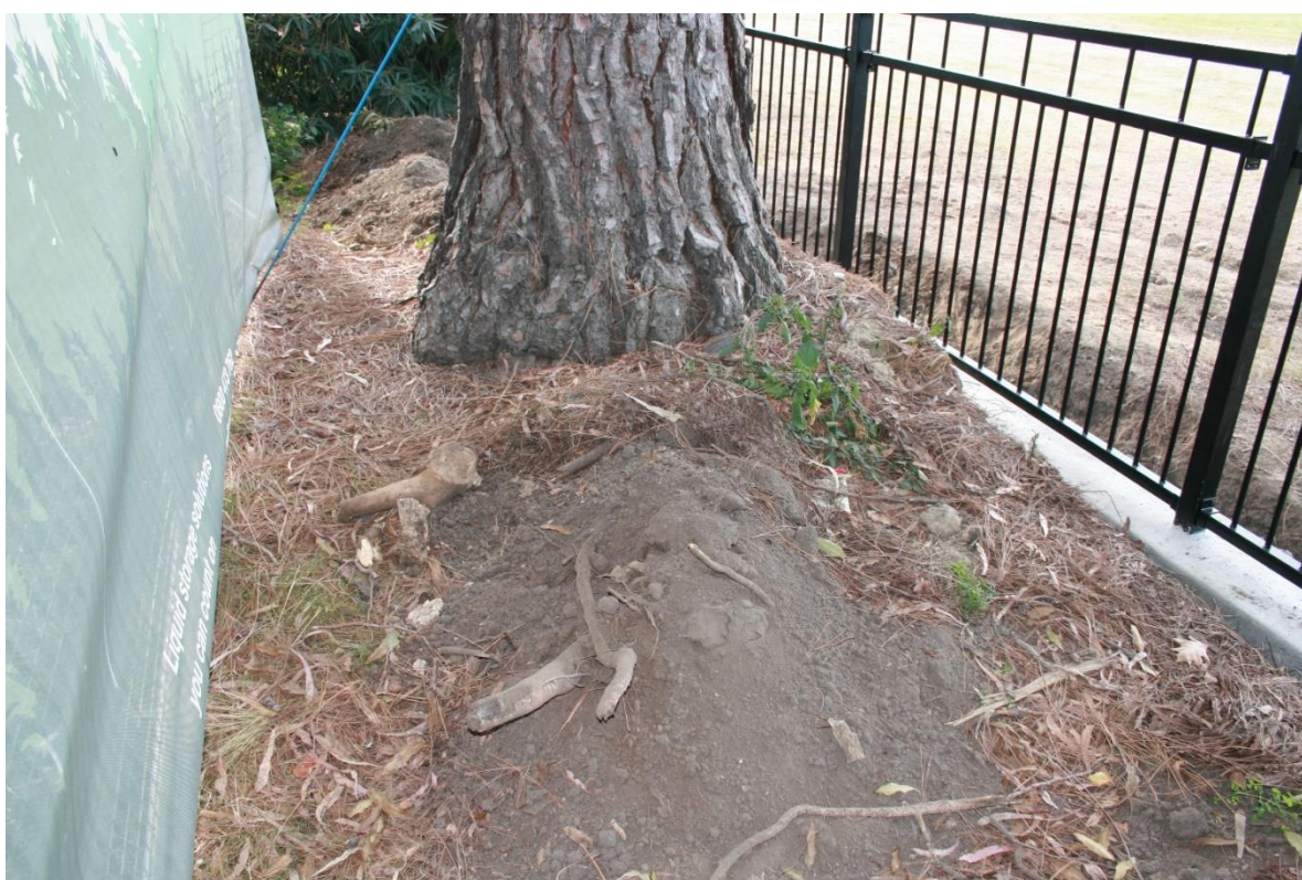
Fig.18 Root damage by contractors installing concrete strip footing adjacent to base of 30m P. ponderosa
