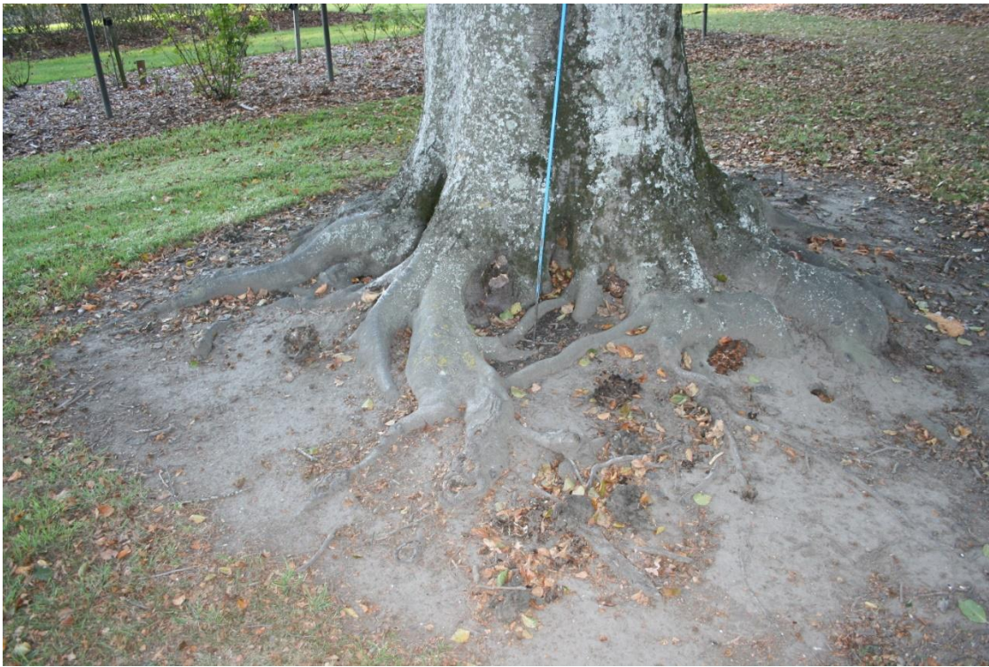
Fig. 7 Area after spraying has occurred, all fruiting bodies killed hiding the significance of the structural loss.
