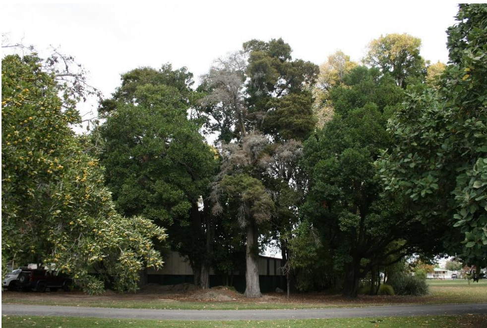
Fig.20 Build-up and scraping of soil at the base of totara, corresponding with canopy dieback
