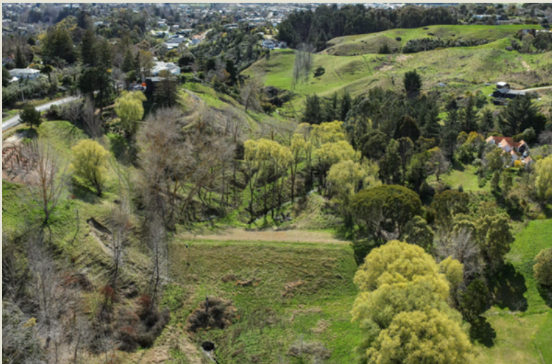
Figure 2: School Dam looking down to Havelock North, with the dam crest (wall) and inlet pipe/ culvert in bottom of photo
