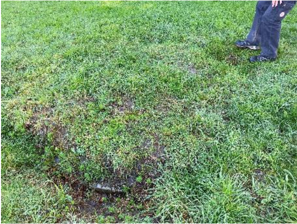
Figure 9-4. Lower: Manhole lid that lifted from culvert water pressure.
