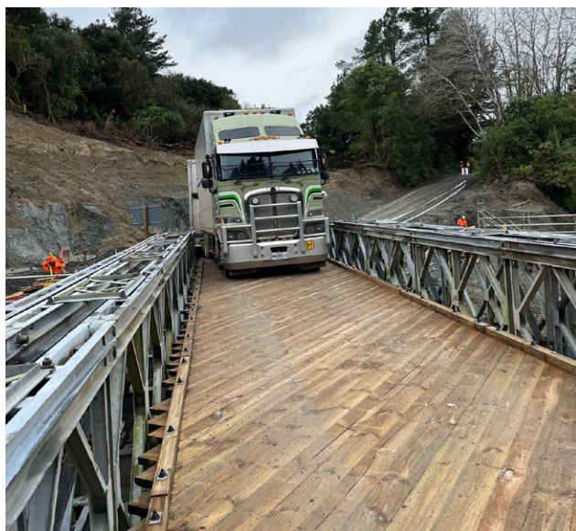
The Mangatutu bailey bridge was opened to traffic on June 15, restoring a vital transport link for the rural community of Waihou. PHOTO/FULTON HOGAN
