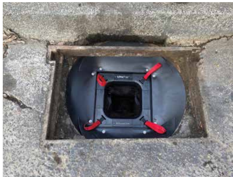
Prototype Littatrap filters being installed in roadside sumps on Hazelwood Street, which drain into Lowes Pit
