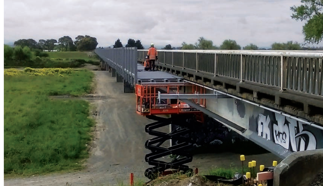
▲ Installation of the Wagner's CFT clip-on pedestrian walkway and cycleway on the Chesterhope Bridge, Hastings.
