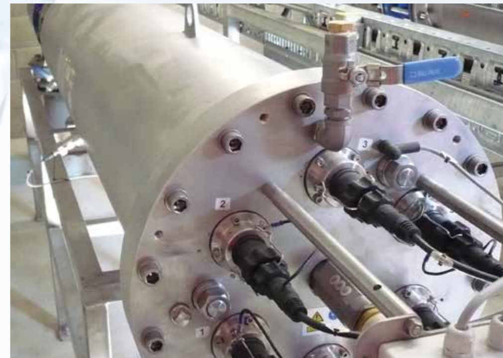
UV disinfection is sometimes used as an alternative to chlorine disinfection. Photo: Queenstown Lakes District Council.
